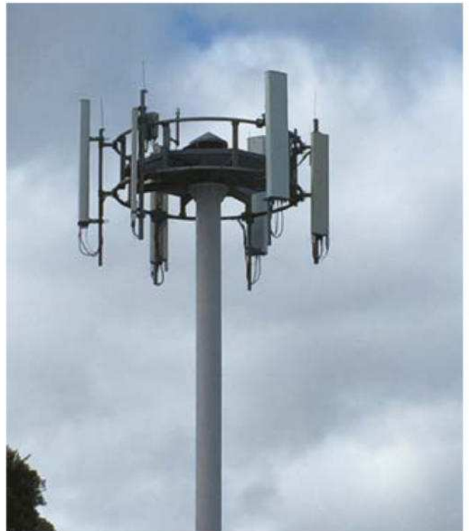
Above: Cellphone tower in a suburban street. With the advent of the 5G network, the proposal is to double the number of cellphone base stations in urban areas. Photo: Katherine Smith
